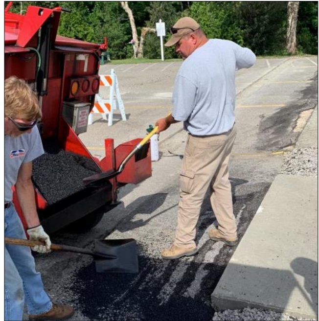
Resurfacing work is under way this month at the Campbell Marine Complex in Georgetown. Workers started repairing pavement at three of our boat launch lanes on July 14. Three of the six lanes will remain open at all times while the other three are resurfaced.
