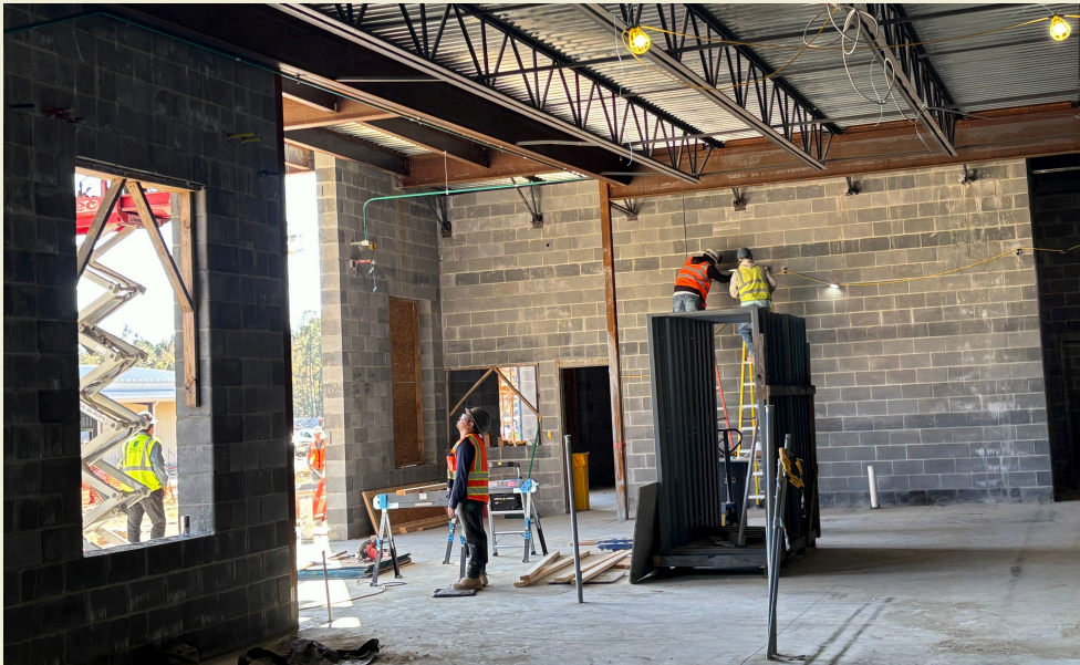
Workers are seen inside the new detention center building under construction on Highway 51.
